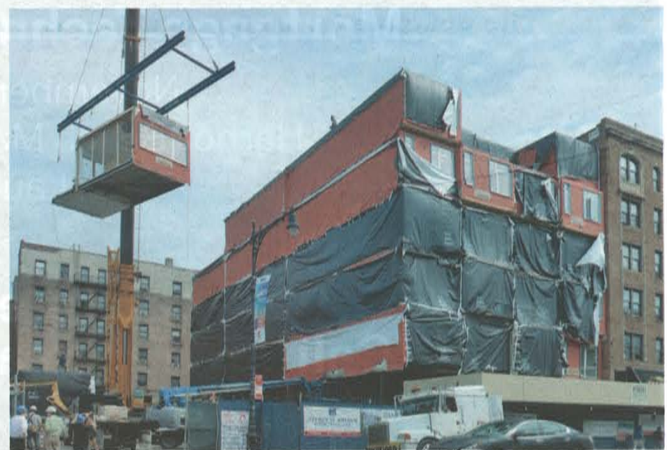
The 45-foot-long moduls for the Inwood building located on the upper tip of Manhattan were constructed in a hangar-size plant in Pennsylvania.
